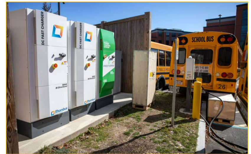
Beverly, MA, uses its electric school buses to sell power back to grid during peak summer days
