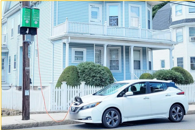
Pole-mounted EV charging stations installed in Melrose, MA, to support “garage orphans”
